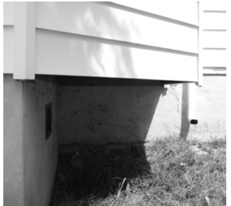
Problem solved: Foundation moved back four feet and part of the addition converted into a ‘architectural projection.’
