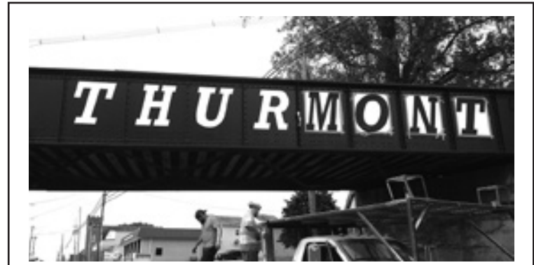
The Maryland Midland Railroad Bridge in Thurmont has successfully undergone the first step in its long overdue rehabilitation. Last month, the Board approved a $25,100 bid by Blackland Industries to clean and re-paint the bridge. The bridge now proudly dons the town's name in big, bold, white letters with a new coat of black paint on the remainder of the bridge.
