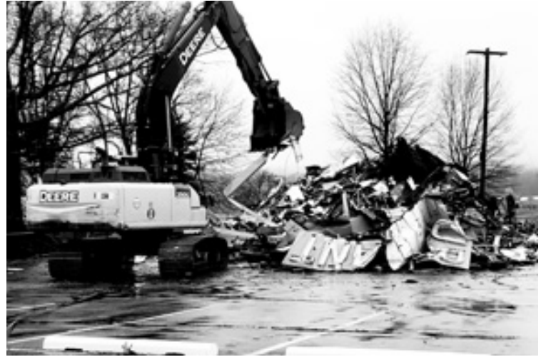
In just a matter of hours, the once proud Shamrock restaurant was reduced to a pile of rubble.
